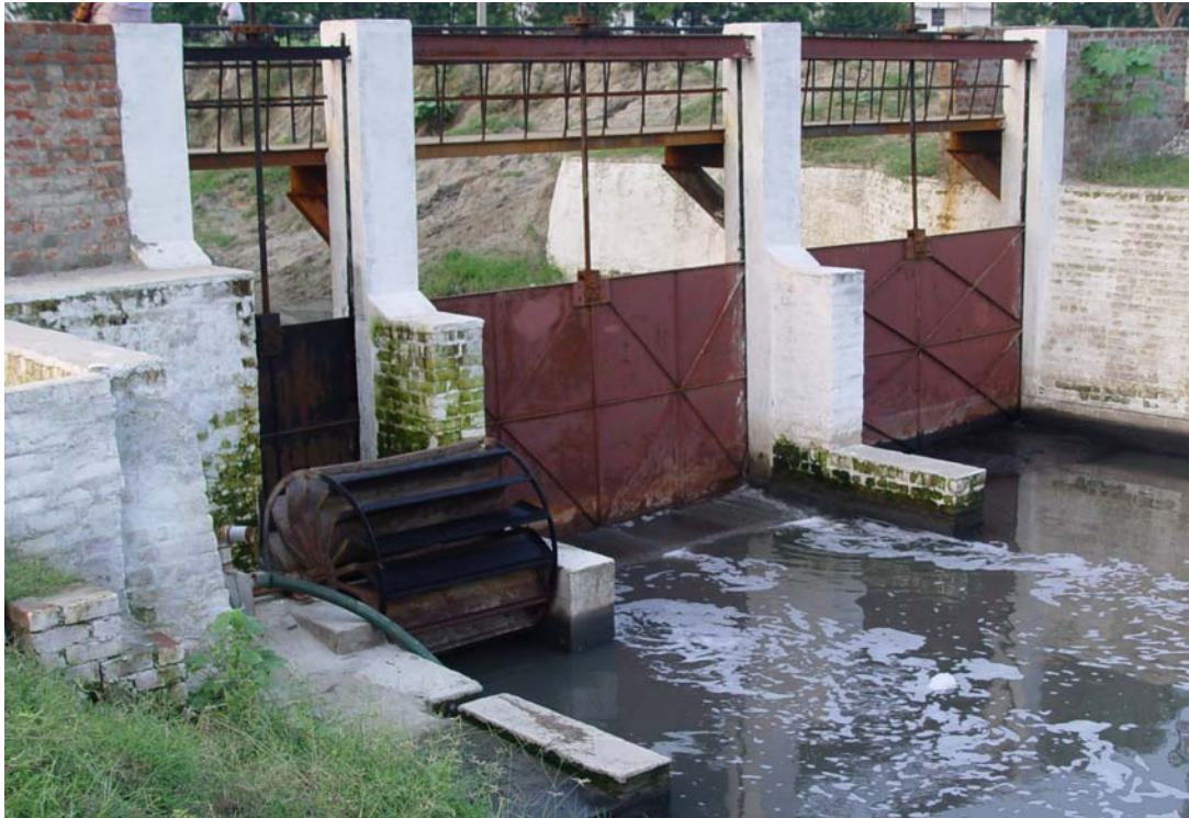
Fig 3. Newly upgraded waterwheel at Sonipat, Haryana, India.
