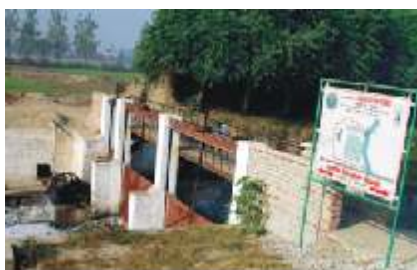
Water wheel installed at Jagdishpur, Sonapat, Haryana on a waste water drain.
